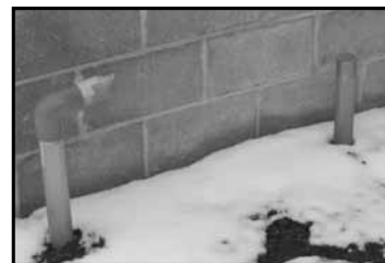
Sawed PVC pipe and missing backflow preventer behind the VGEM entrance wall
