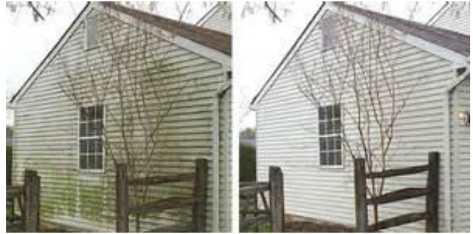
Mold on house exterior on left and after power washing on the right
